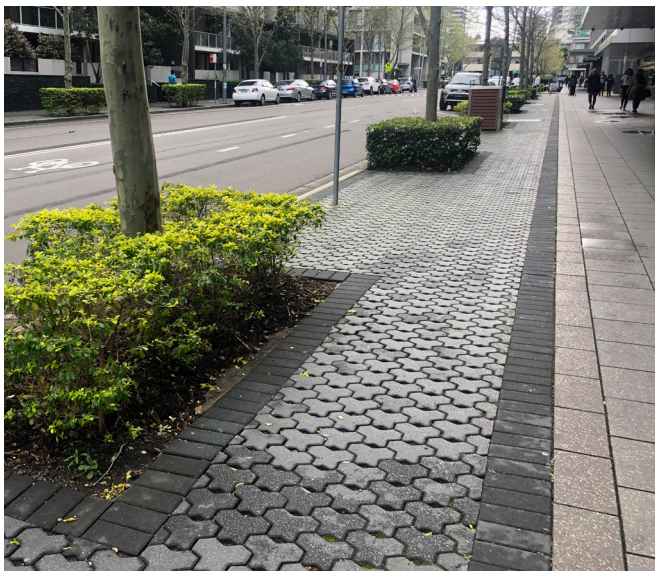
Permeable paving for street trees on Rider Boulevard, Rhodes. Image - (ASPECT Studios)
