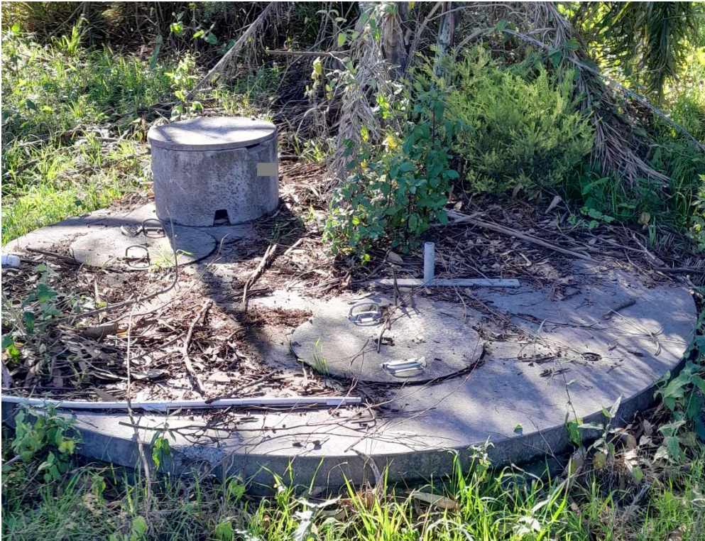
Example of a poorly maintained and overgrown AWTS tank
