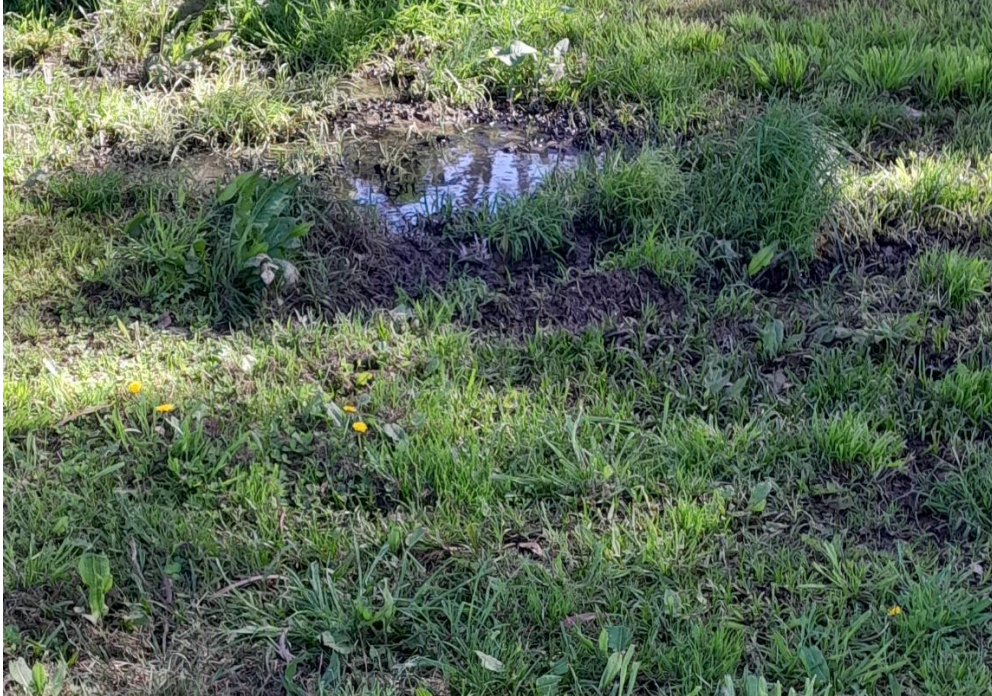
Example of a failed AWTS irrigation sprinkler system (ponding of effluent)
