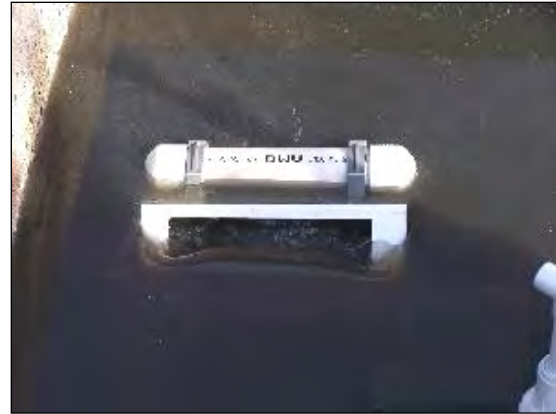
Figure 14.7 The Flout® reaches the maximum level in the chamber
