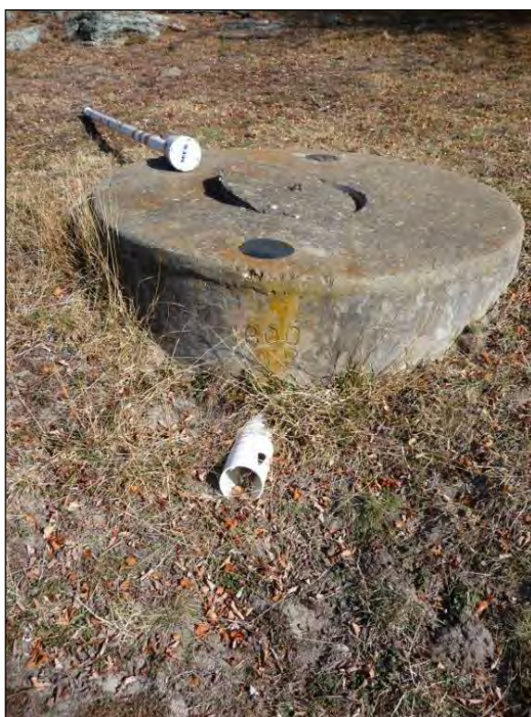
Figure 3.7 Outlet pipe discharging directly onto open ground
