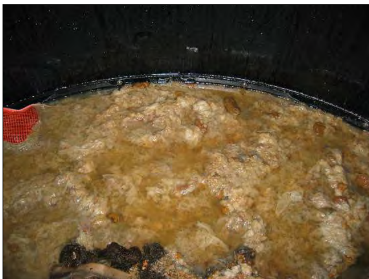
Figure 5.9 A flooded system due to pump failure
