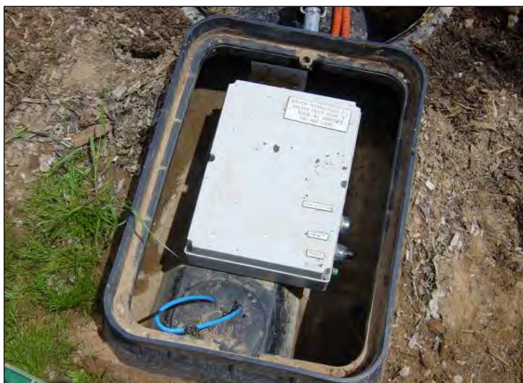
Figure 5.8 An electrical box that was flooded
