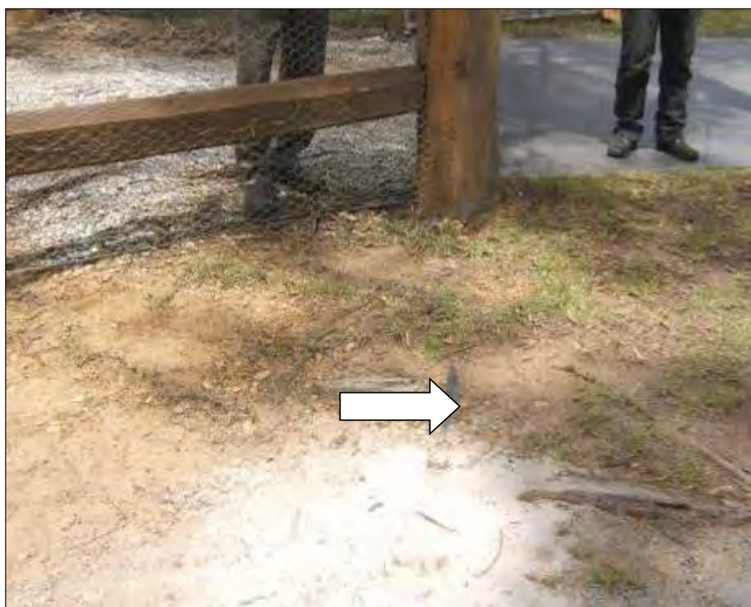
Figure 2.2 Main irrigation line buried at only 50mm under gravel driveway – 500mm is the minimum required depth.
