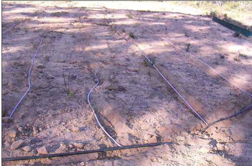
Figure 13.7 Poorly installed subsurface effluent irrigation system
