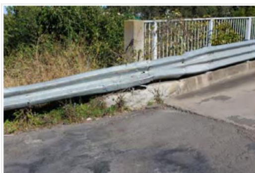
Plate 6 - Impact damage to rail and kerb
