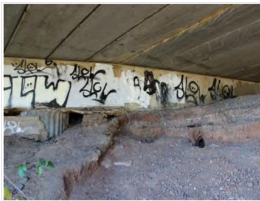
Plate 4 - Erosion below abutment
