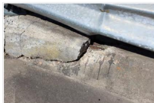
Plate 7 - Cracked kerb with exposed reinforcement
