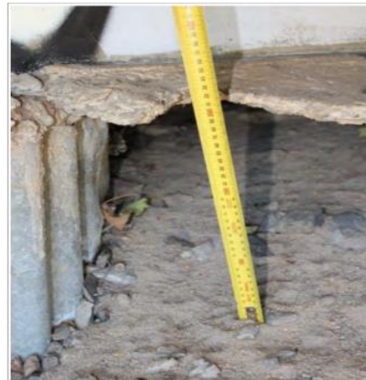
Plate 5 - Depth of erosion (300mm)
