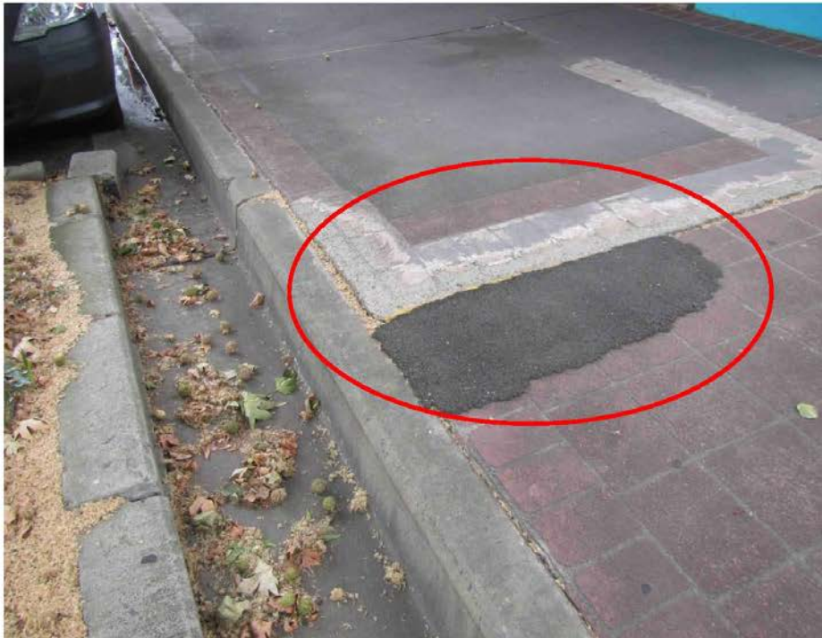
Figure 12 Shows more raised concrete that has been shaved to reduce tripping
