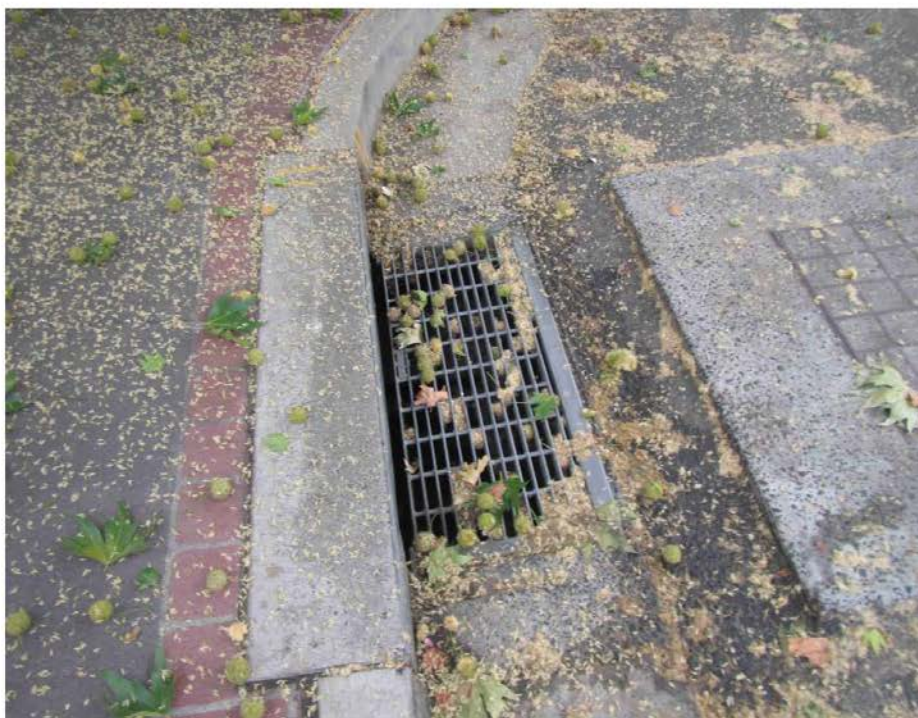
Figure 8 Shows a street drain that would get covered by leaves and seed balls
