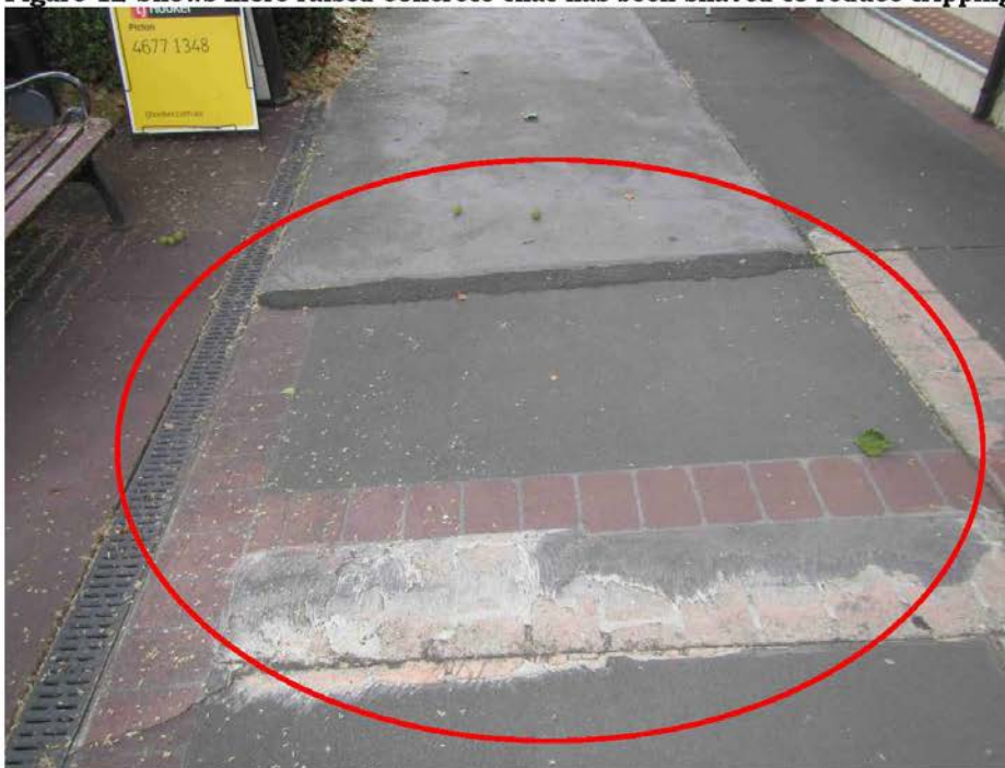
Figure 13 Shows again trip hazards from lifting concrete.
