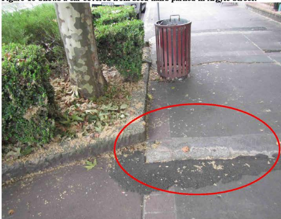
Figure 11 Shows raised concrete that presents a major trip hazard.
